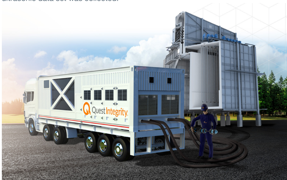
Figure 3. Typical Fired Heater Set Up for Advanced Cleaning and FTIS Inspection
